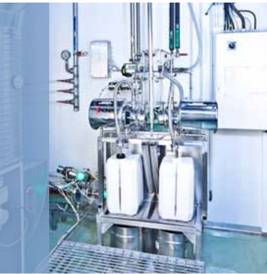
Clean in Place – Station (CIP)
